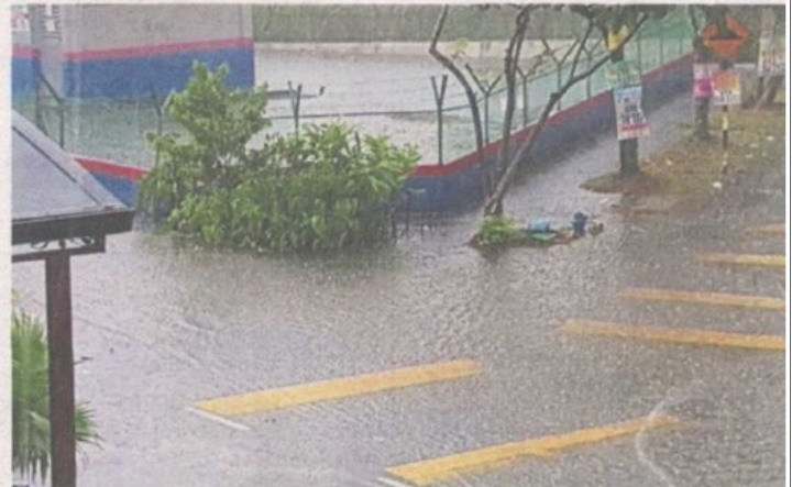
Water overflows into the compound of the TNB substation in Taman Sri Manja every time it rains.
